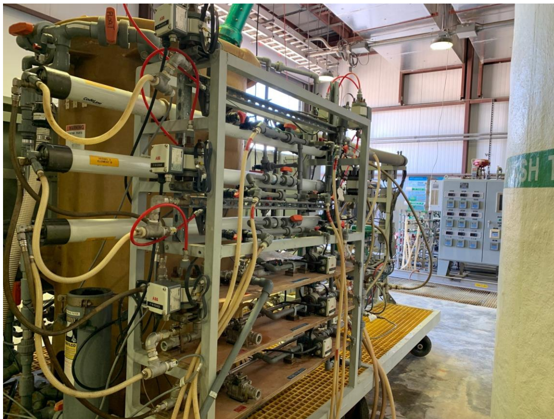
Fig. S8. Image of the element screening unit at the Yuma Desalting Plant. Pictures are the three pressure vessels with two membranes each. The top two pressure vessel are the first stage in series. The last pressure vessel is the second stage. The high pressure pump (not pictured) is used to feed the brackish water from the feed tank to the first stage pressure vessels.
