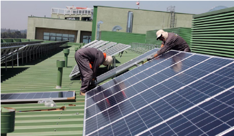
A public hospital in Chile generates electricity with solar panels. Photo: Complejo Asistencial "Víctor Ríos Ruiz".
